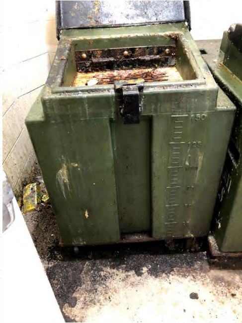
Spillage and absorbent around tank, no signage.
